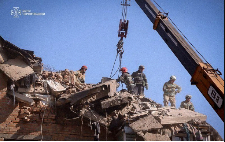
Rescuers on the rubble with the crane
