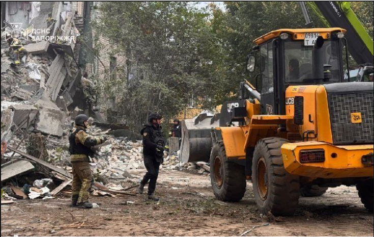
Rescuers and machinery at the destroyed residential building, Zaporizhzhia
