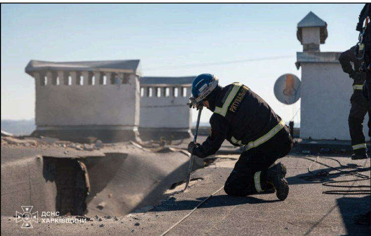
The hole in the roof left by the strike State Emergency Service of Ukraine (DSNS) · 2026-10-12 · CC BY 4.0 https://t.me/dsns_telegram/77419
