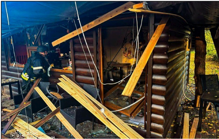
The damaged café in the park
