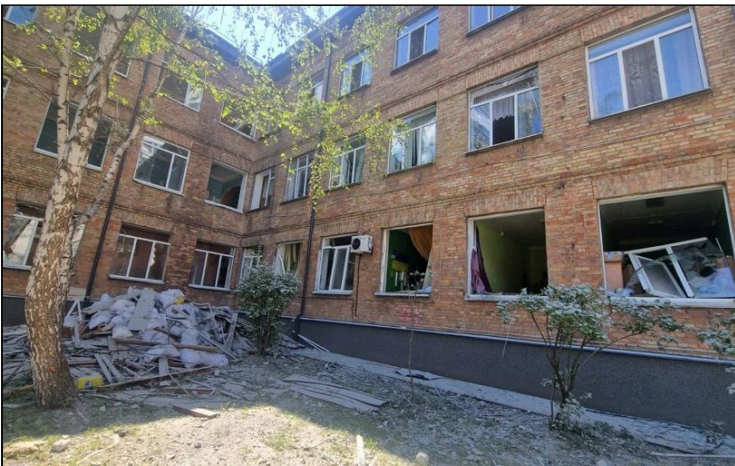
A school building damaged the same night
