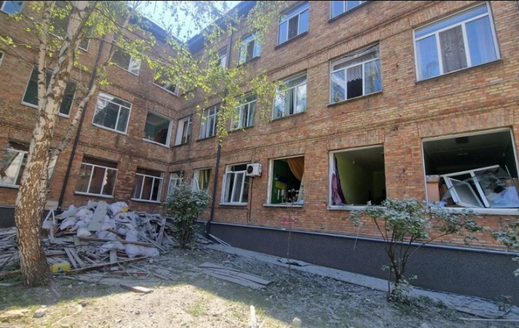
同一夜受损的一座学校建筑 Kyiv City State Administration · 2026-07-02 · CC BY 4.0 https://commons.wikimedia.org/wiki/File:Destructions_in_Kyiv_after_Russian_attack_2026-07-02_(50).jpg
