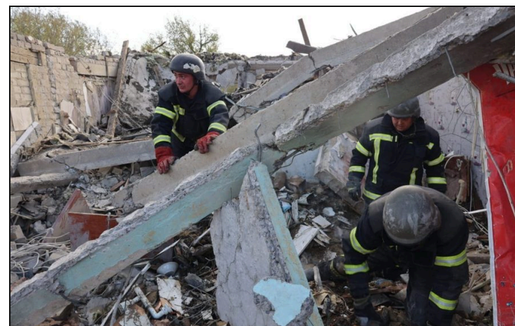
Rescuers work among the collapsed slabs of the building
