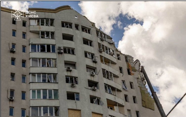
The 16-storey block after rescue work ended
