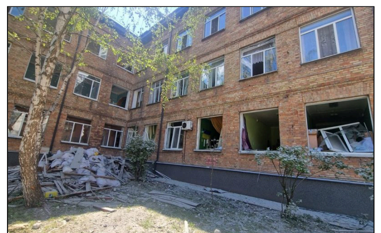
A school building damaged the same night
