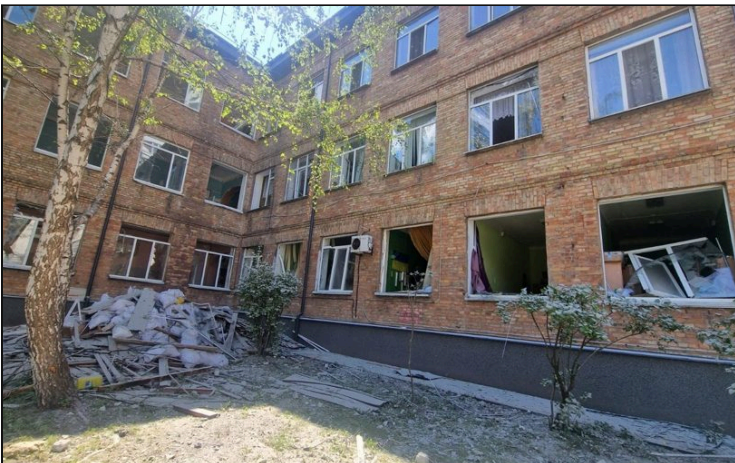
A school building damaged the same night
