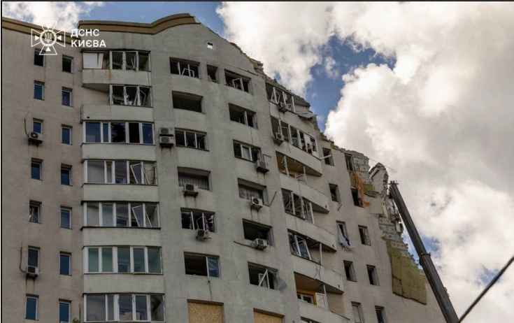
The 16-storey block after rescue work ended
