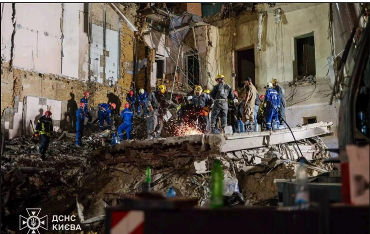
Volunteers pass debris hand to hand at the hospital
