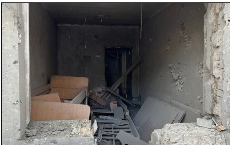
A damaged ward of the hospital
