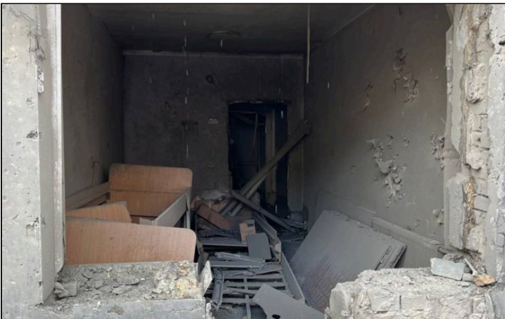
A damaged ward of the hospital
