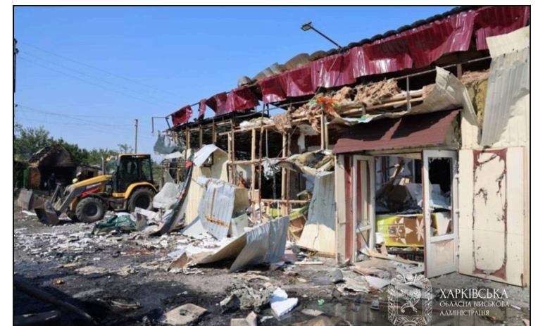
The centre of Pechenihy after the missile strike of 18 August 2026 — regional administration release, frame 6 of 6
