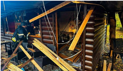
Nova Vodolaha: the site after the strike · State Emergency Service of Ukraine (DSNS) · 2026-10-19 · CC BY 4.0
